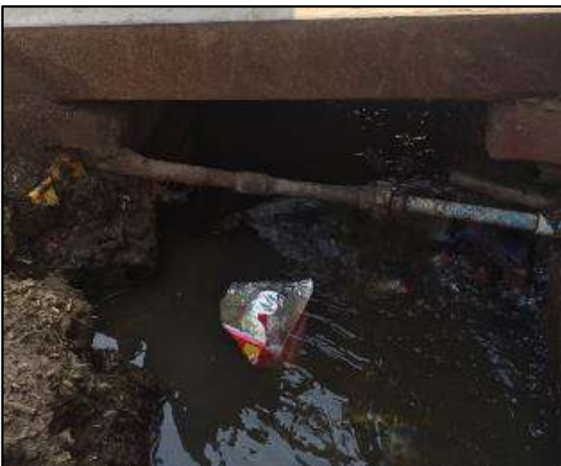
Pic.1: Water leakage from rusted pipe line
