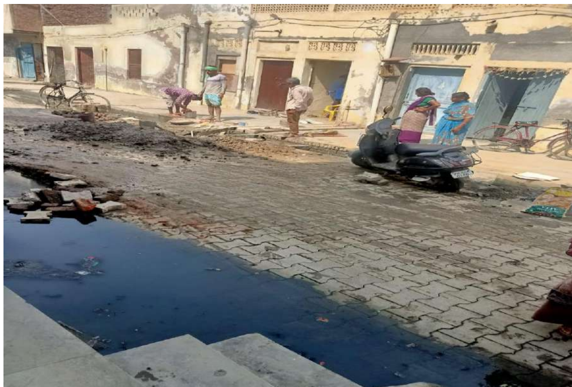
Figure 3: Reverse flow from gutters (Photo 2)
